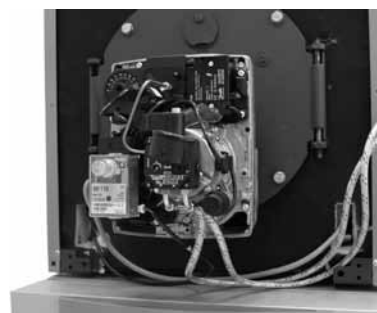
Cable run burner - boiler
